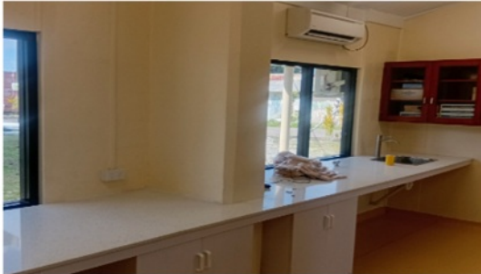
Renovations supported by the KOICA SHAPE project for the Food, Water, and Leptospirosis MAT Laboratory at the Fiji CDC
